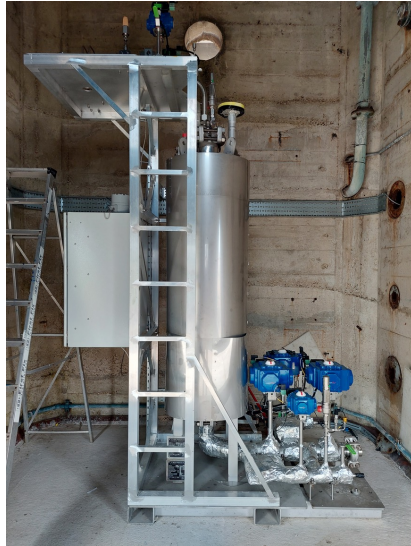
(a) LOX high pressure skid
