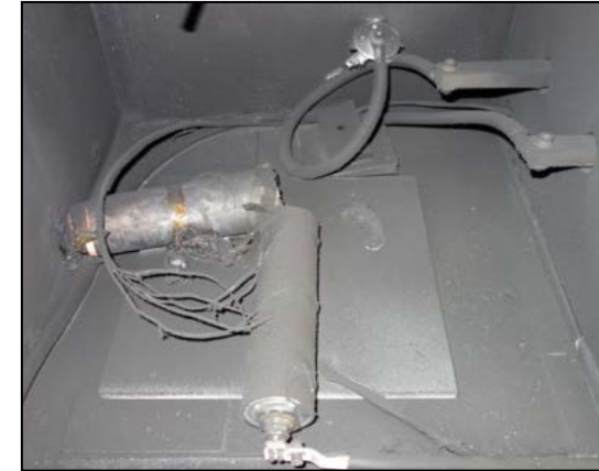
3 mΩ short-circuit on VES140
