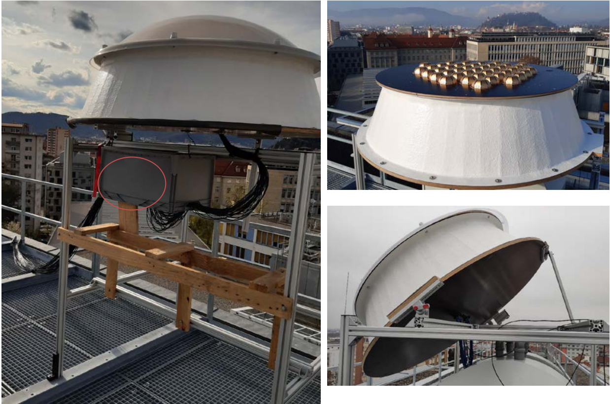
Figure: Left: AP antenna array carrier. The low-loss antenna cables from the array are going to the sampling units. Upper right: plate with 40 antennas. Lower right: possibility to tilt unit.
