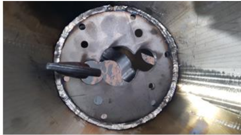
Full Penetration weld as corrective action for endcap popping off on Inconel Cones Project 4
