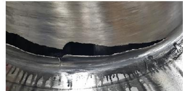
Close up of the right end crack propagation
