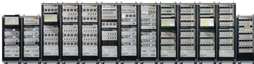
Figure 2-1: Example of Rovsing turn-key Power SCOE
